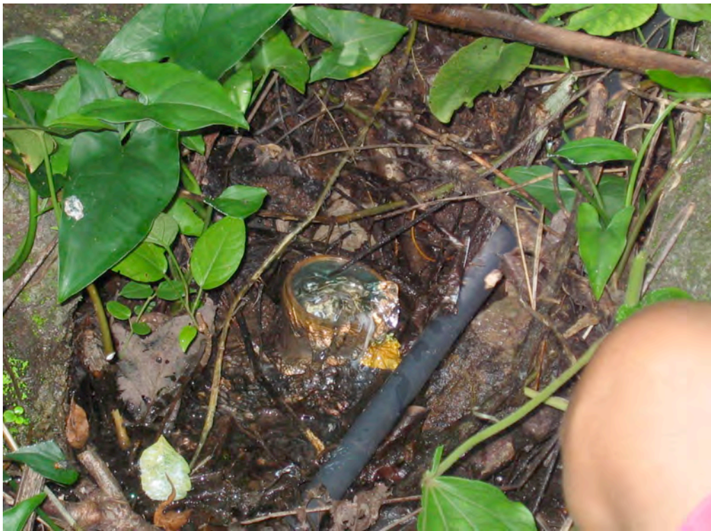
Two photos of decay, disrepair, and the potential for disease: in the top photo, leaks in the captation tank and hoses attempting to recapture leaking water; in the bottom photo, a dead rat is stuck in the pipe that supplies water to the people of El Zapote.
